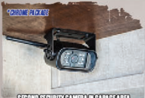
SECOND SECURITY CAMERA IN GARAGE AREA
