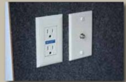
110v Outlet and Cable Hook-up in Pass Thru Storage Area.
